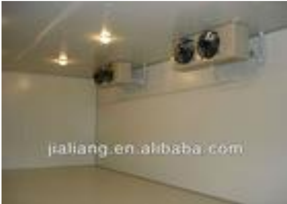
Interior view of typical cold room
